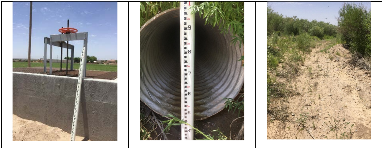
Figure 7. Photographs showing the irrigation turnout (left), 36" culvert (center), and excavated irrigation canal.
