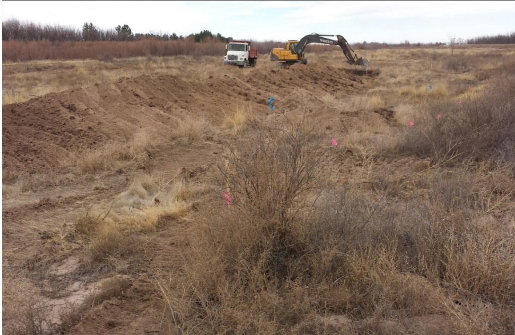
Figure 3.3. A swale is excavated by removing the top several feet of soil to lower the soil surface elevation. Removed topsoil is trucked to spread on nearby roads. Note native wolfberry shrubs flagged to avoid damage or disturbance (Main Swale, Berino East).
