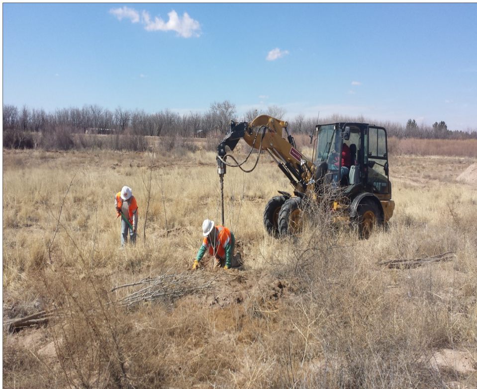
Figure 3.5. Restoration crew planting cottonwood poles into intact native grassland using a frontloader-mounted auger (Grassland Auger Area, Berino East).
