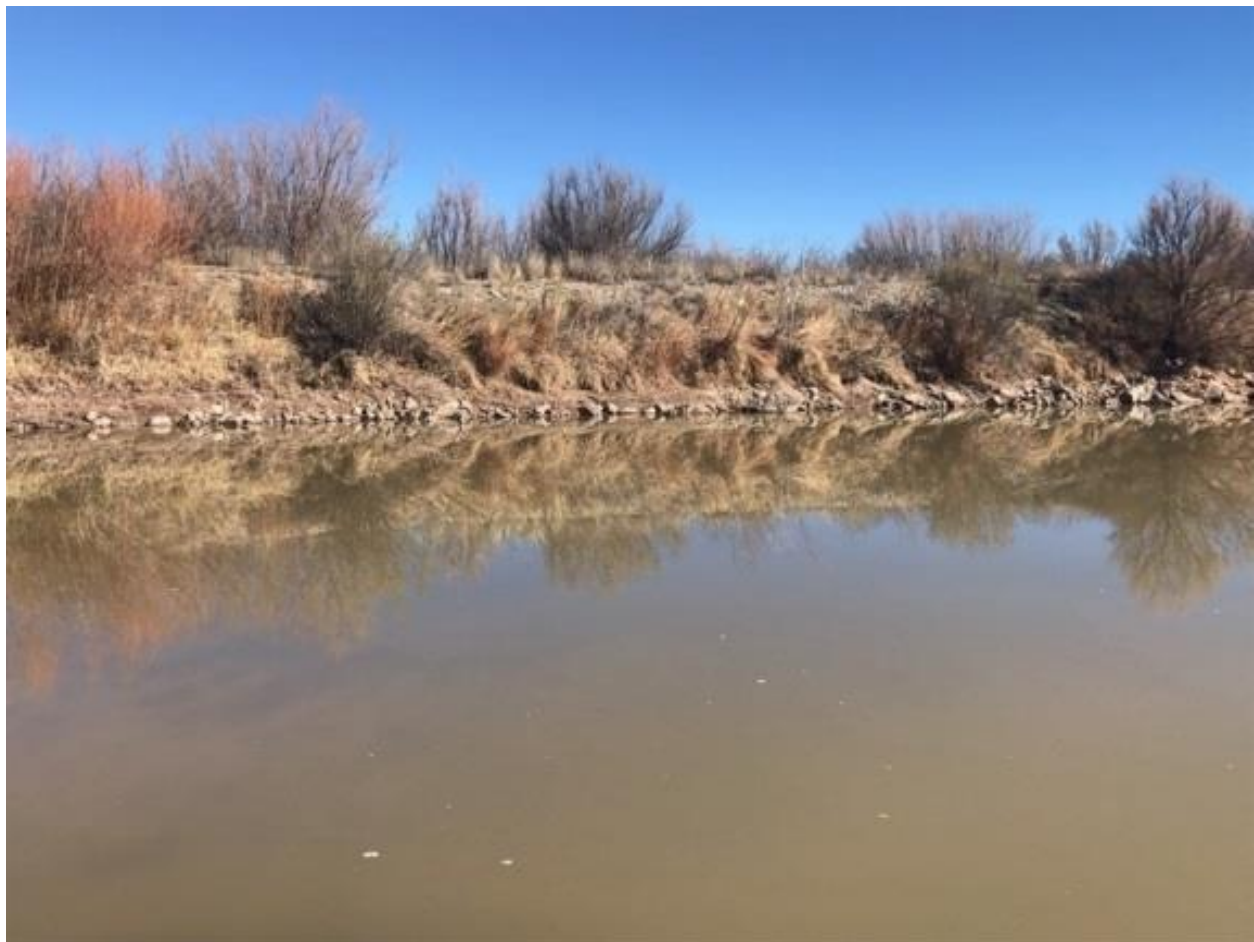
Photograph 2-1. Riprap along the toe of the bank at Yeso Arroyo Alternative site
