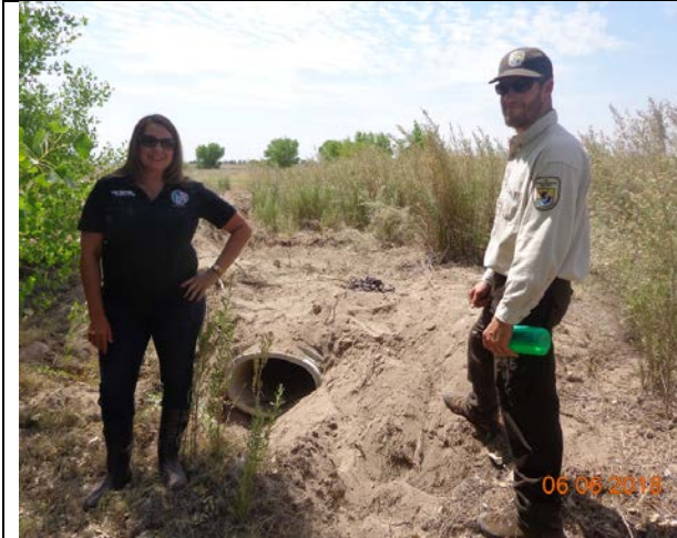
USFWS and USIBWC check out the new pipe connection to the new irrigated cell, June 2018
