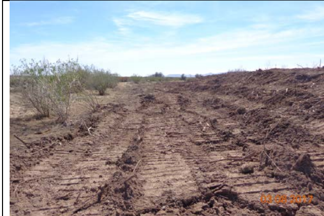
Excavation work includes lowering the inset floodplain by several feet. Contractors hauled away over 5,000 cubic yards of material, March 2017
