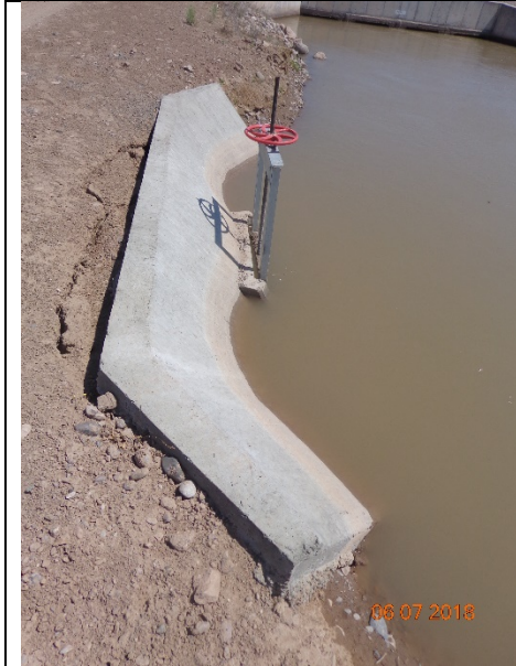
Check structure at Garfield Lateral to constructed by EBID in April 2018 to irrigate Crow Canyon B site.
