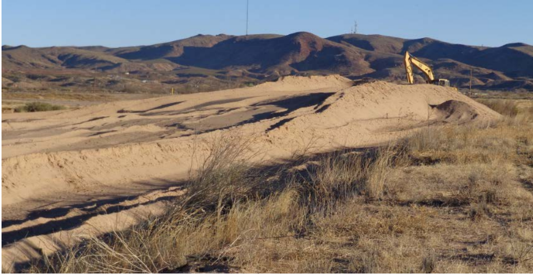
Figure 38 USIBWC crews create a temporary sediment stockpile in the floodplain of excavated sediment near Rincon Arroyo, March 2014
