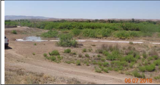
The connection between the check and the irrigation piping leaked some water, and USFWS fixed the leak the following week. The water was still beneficial to the plantings near the siphon. June 2018
