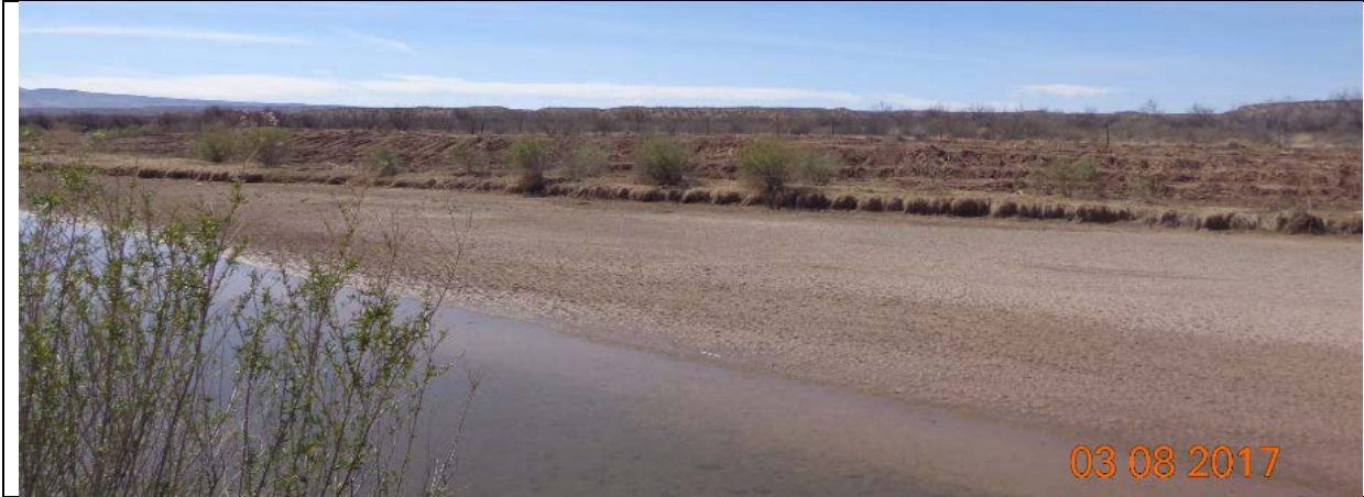
View of the site from Yeso East after saltcedar removal and initial excavation, March 2017.
