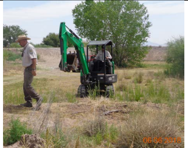
USFWS prepare to fix gopher holes in the irrigation berm to prevent leaks, June 2018
