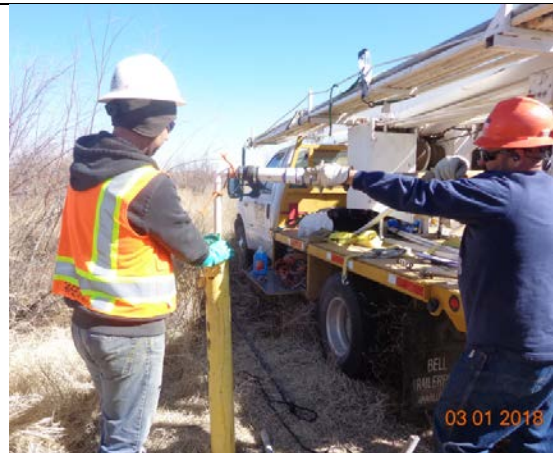
USIBWC well contractor EGC is rehabbing well at Vinton B and retrieving the sonde from the well, March 2018.
