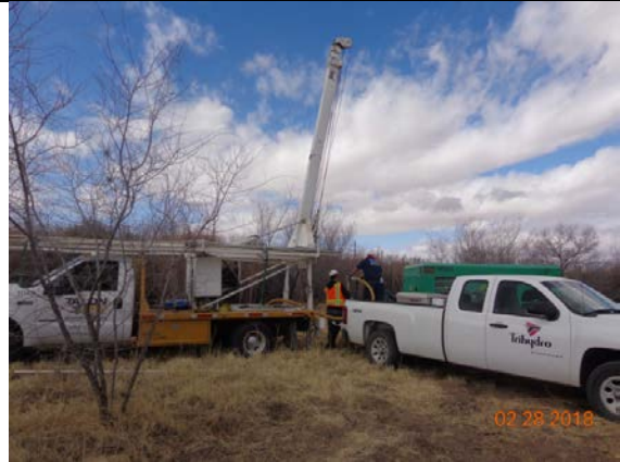
Contractors EGC and their subcontractors conducting well rehab by removing sand obstruction in AB-MW-2, February 2018.
