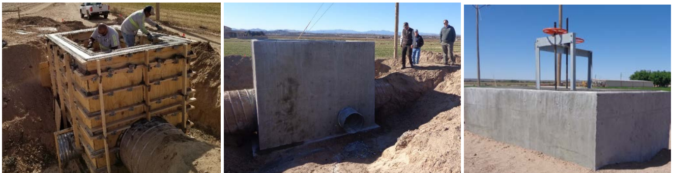
Figure 27. Left: EBID constructing a box at Trujillo Lateral in Dec 2018. Middle: Site visit of the structure with USFWS and EBID in late December 2018. The structure will allow irrigation of the Trujillo site in 2019. Right: completed structure May 2019.
