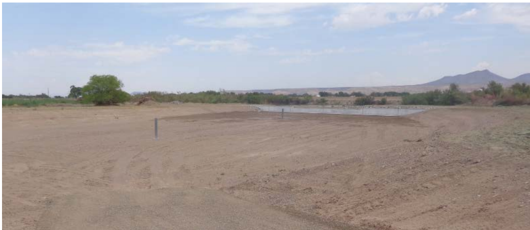
Figure 37 Thurman I Sediment Basin after construction and after a storm event June 2019
