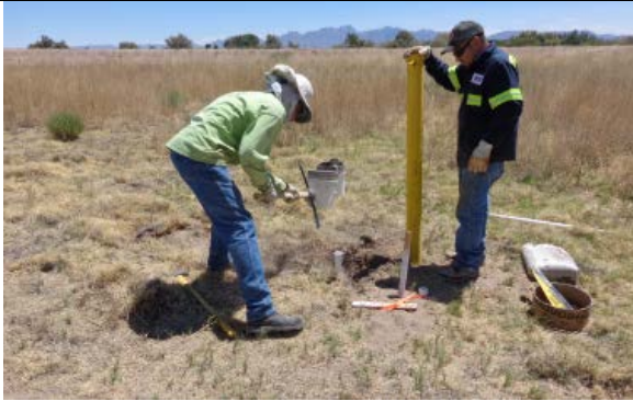
In 2013 and 2014, USIBWC contractors constructed 55 groundwater monitoring wells at restoration sites throughout the Rio Grande Canalization Project. Here, contractors cap a well at Mesilla East June 2013
