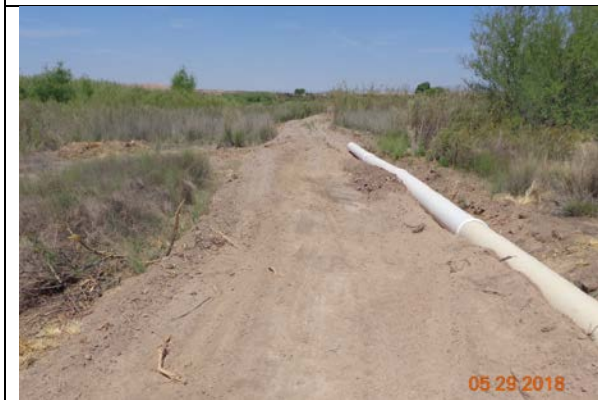
USFWS installed 12" irrigation piping to deliver the water via pressure against gravity to the site upstream of the Garfield Lateral turnout.
