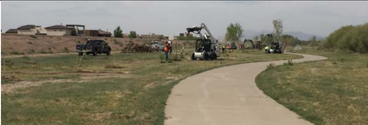
Teams of equipment operators planting cottonwoods and Gooddings in clusters along the recreational path, using both auger and trench methods, April 2018. This site is a park maintained by City of El Paso.
