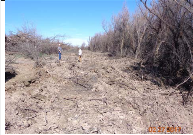
Contractor has begun removing a large swath of saltcedar. Contractors/ USIBWC meet to discuss excavation work, Feb 2017
