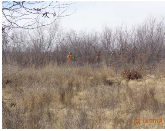
Chainsaw crews are slowly working through the 35 acres at Vinton A and B removing saltcedar, March 2018.
