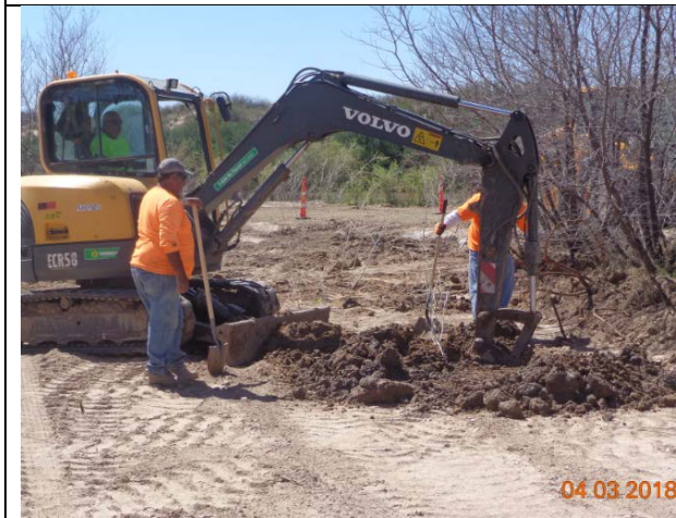
IDEALS crews planting cottonwoods and Gooddings in the excavated swales with trenches, April 2018.
