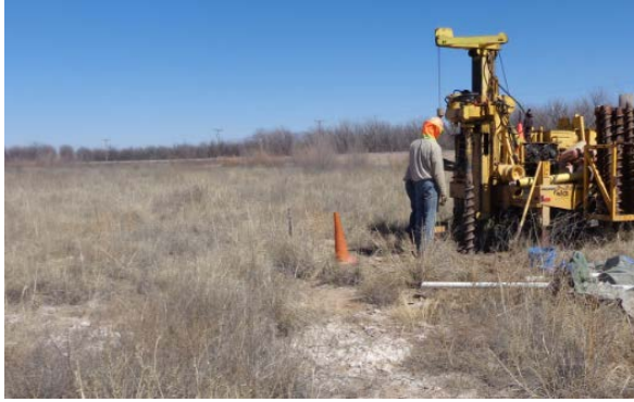
Contractors redrilled groundwater monitoring well that was obstructed at Berino East, March 2018.
