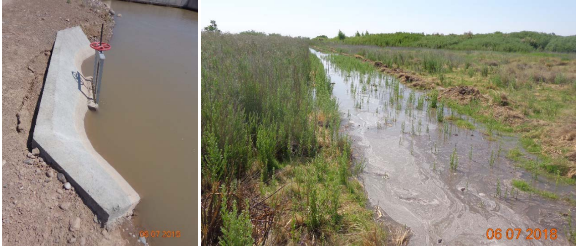
Figure 24 (Left) Check Structure at Garfield Canal built by EBID in April 2018 to irrigate Crow Canyon B; (right) Irrigation of Crow Canyon B via irrigation piping and then earthen V-ditch in June 2018
