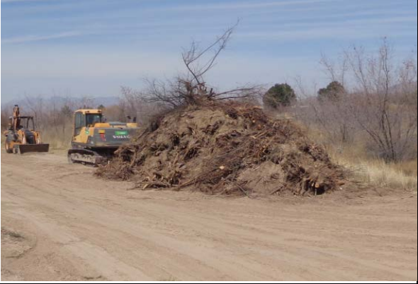
Piles of saltcedar debris along the levee road will later be hauled off, March 2018.
