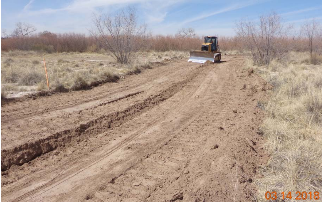
Figure 12 Excavation of swales at Country Club East by USIBWC Contractor IDEALS-AGEISS, March 2018
