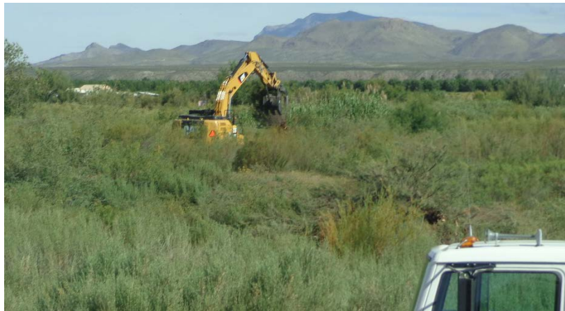
Figure 31 USIBWC Las Cruces Field Office crew removing saltcedar with an excavator in a No Mow Zone on the west floodplain north of Hatch, NM, September 29, 2016
