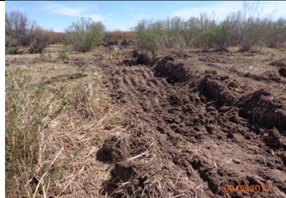
Two inlets were created to allow high flows to enter the site, March 2017
