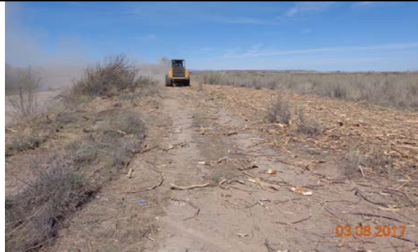
Masticator mulching the saltcedar along an old road near the riverbank, March 2017
