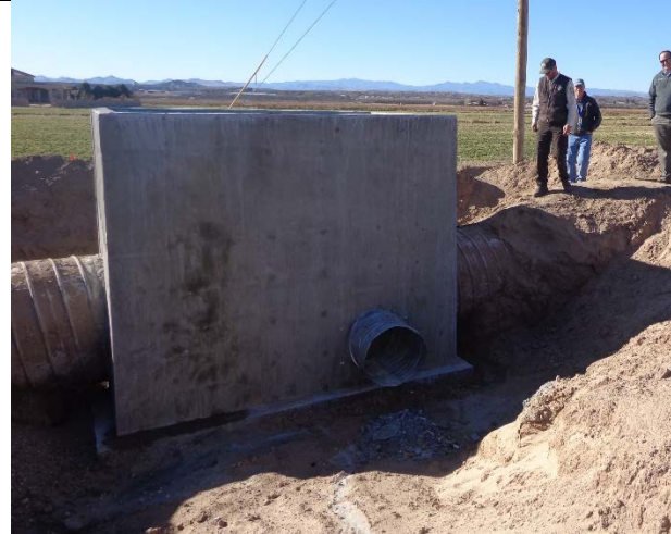
Site visit of the structure with USFWS and EBID in late December 2018. The structure will allow irrigation of the Trujillo site in 2019.
