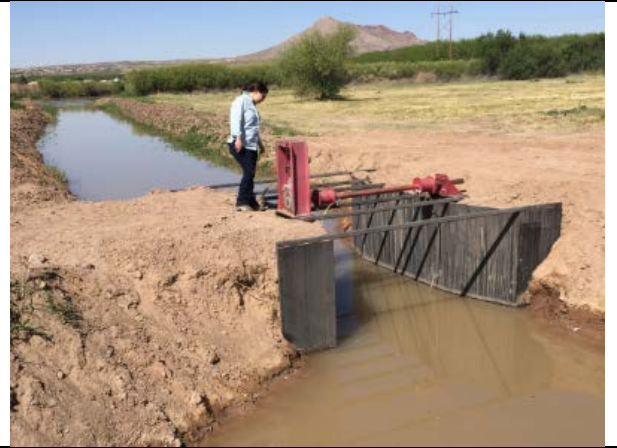
EBID constructed a new turnout structure at WW 8 for USIBWC to irrigate this site. April 2017.
