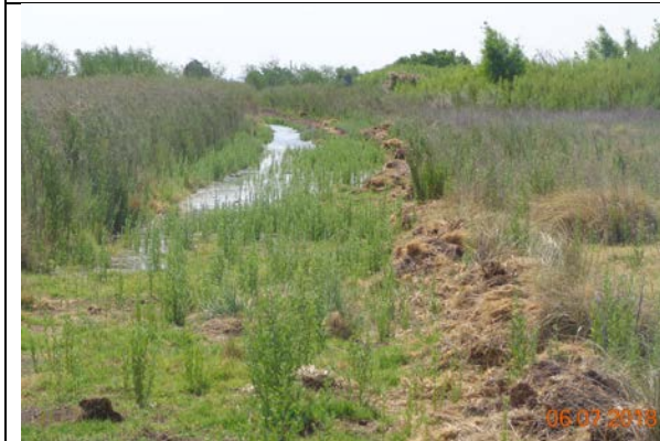
The piping system was continued by an earthen V-ditch throughout the site.
