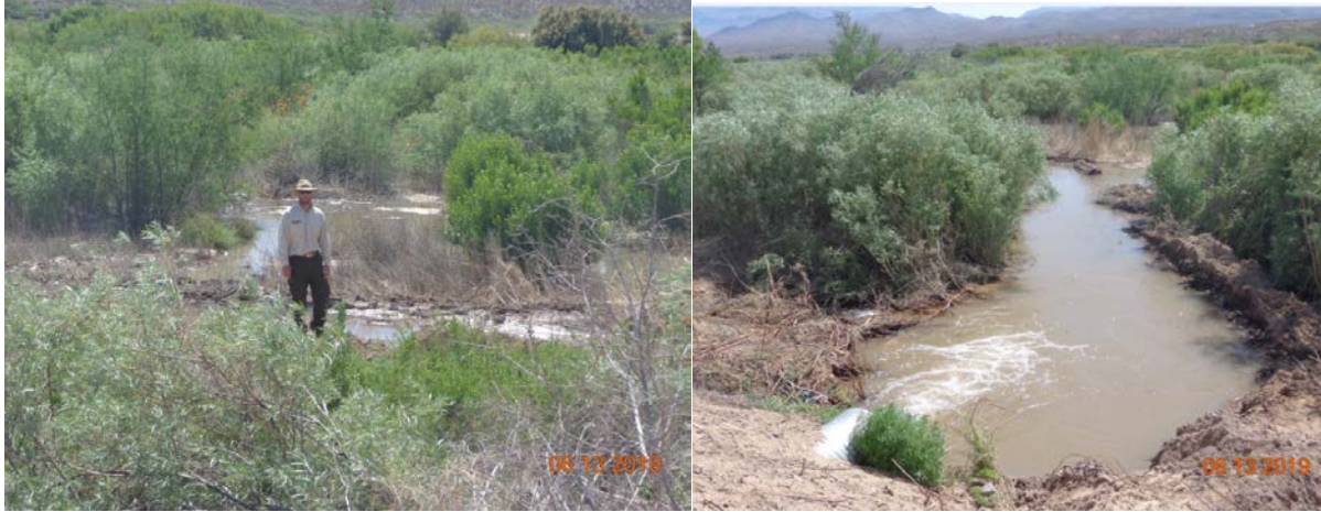
Figure 28 Trujillo Restoration Site first irrigation event June 13, 2019. Left: Tyler from USFWS inspects the earthen diversion channel that USFWS constructed throughout the northern part of the site; Right: water gushes into the restoration site from the pipe connected to the Trujillo Lateral.
