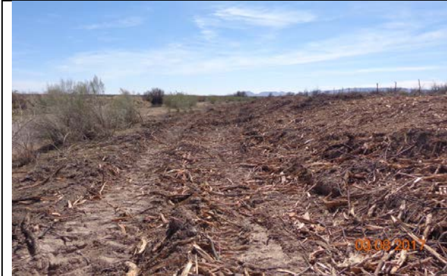
Saltcedar was masticated on site at the northern end of the site to prevent erosion from high flows, March 2017
