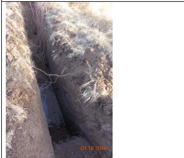
Willows are transplanted into excavated trenches which hit the groundwater table. At Anapra, this was about seven feet below surface. January 2018.
