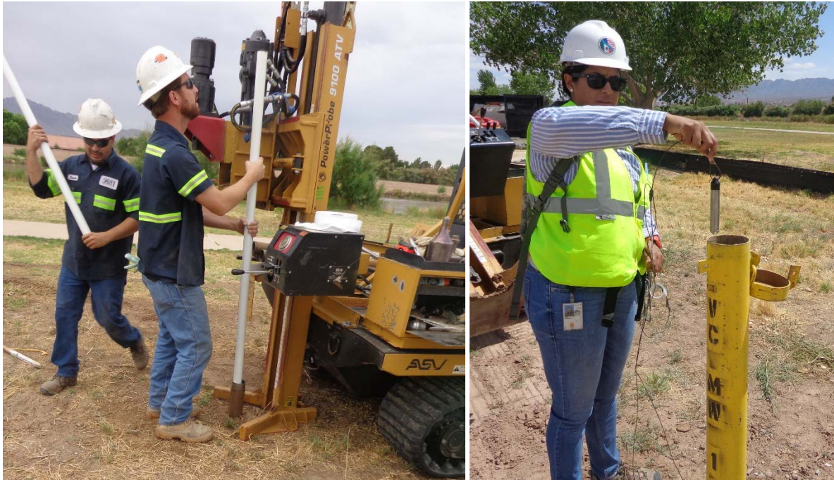
Figure 17 Drilling and installing a groundwater monitoring well at Valley Creek in July 2014 (Left); USIBWC's Nereida Cora deploying an automated logger in the new well (right)
