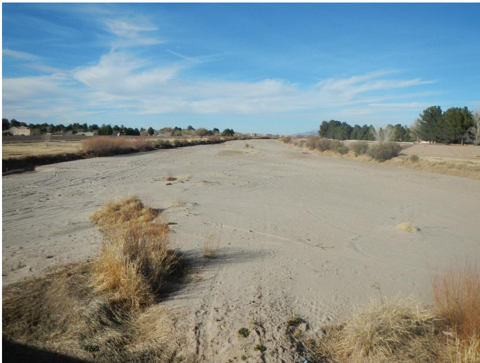
Photo A.74. View upstream from Country Club Bridge showing the intermittent grass and light brush vegetation along the banks.
