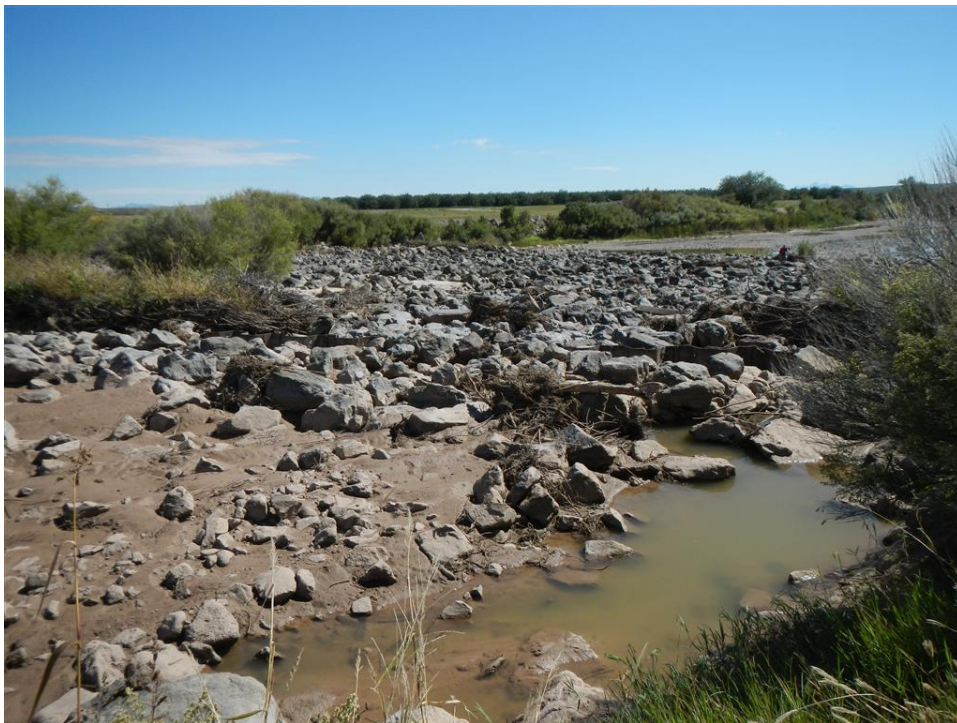
Photo A.28. View downstream along the rock riprap and sheetpile grade control structure for the Rincon Siphon.
