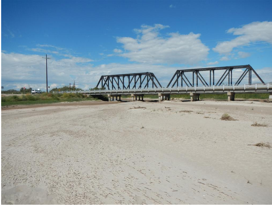
Photo A.27. View upstream to the New Mexico Highway 154 Bridge at the Problem Location 3 site. Also shown is the BNSF Railroad Bridge in the background.
