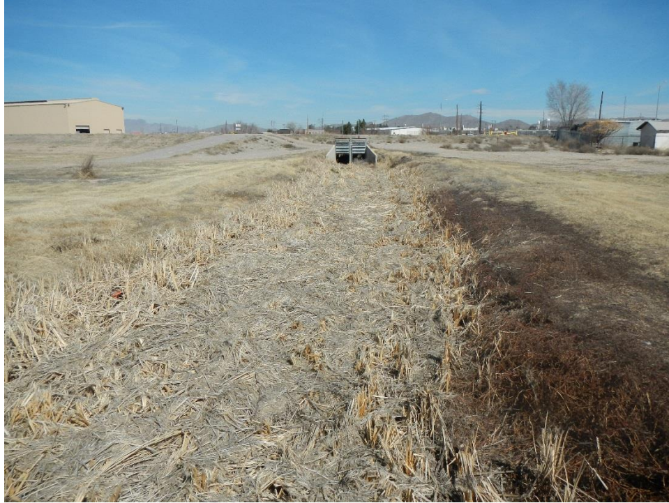
Photo A.66. View upstream along the lower end of the East Drain to the control structure.
