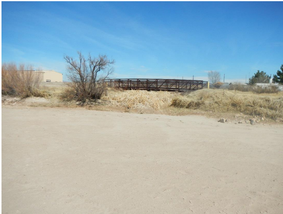
Photo A.65. View to mouth of the East Drain where the bed of the drain has become overgrown with cattails.
