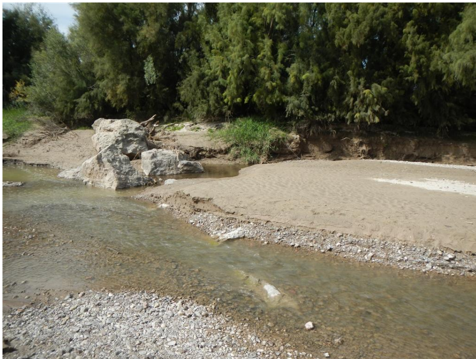
Photo A.2. View along the right bank crest portion of the Tierra Blanca Vortex Weir. Note the sediment deposition along the portion of the weir in the main channel.
