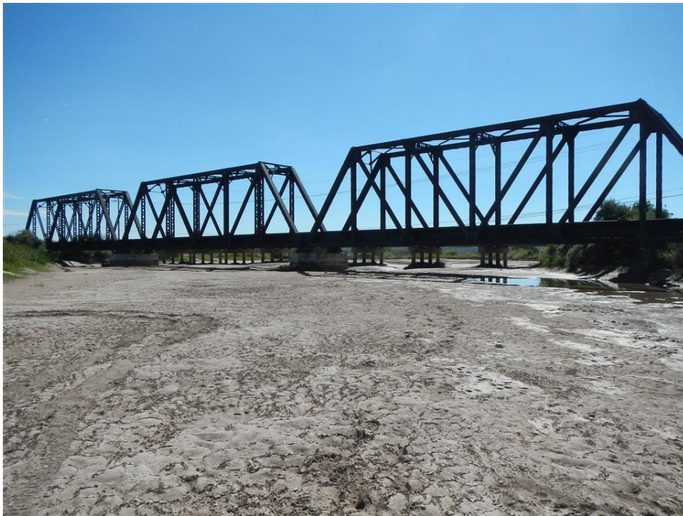
Photo A.26. View downstream to the BNSF Railroad Bridge at the Problem Location 3 site.
