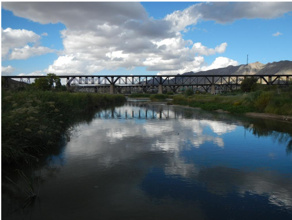
Photo A.80. View upstream to the pair of Southern Pacific Railroad Bridges above American Dam.
