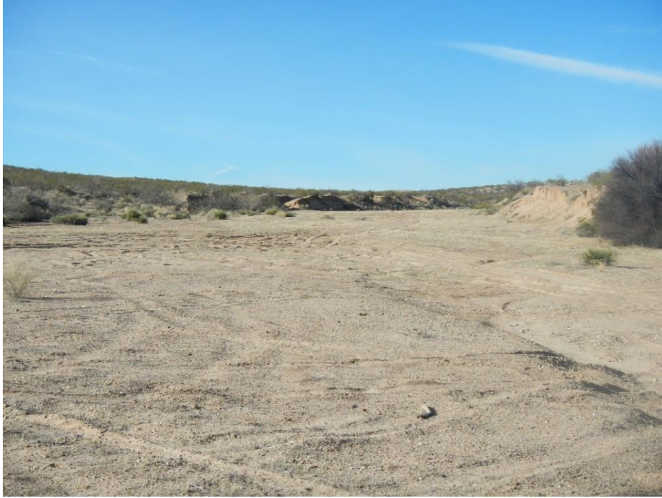
Photo A.59. View upstream to the largest of the right (west) bank arroyos at Problem Location 6.
