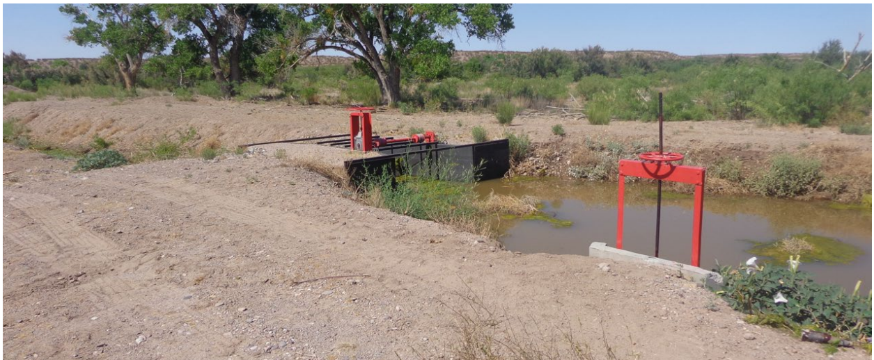
EBID built a turnout at Palmer Lateral in 2019 to irrigate the Yeso East site.
