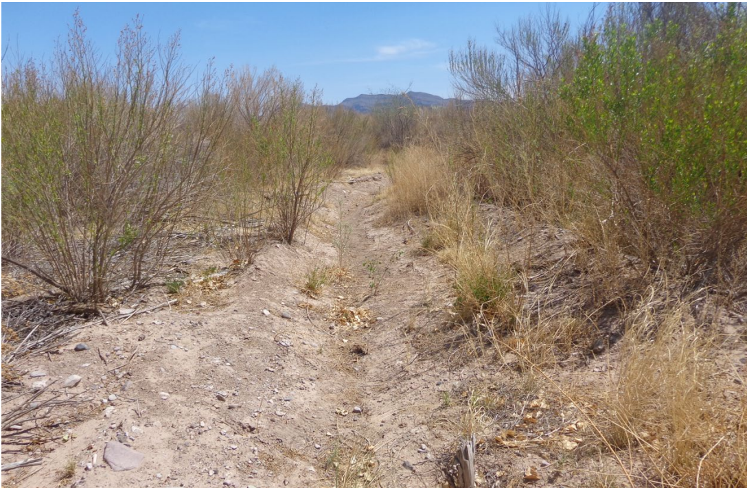
Earthen v-ditch that conveys water upstream of the turnout, prior to water reaching it.
