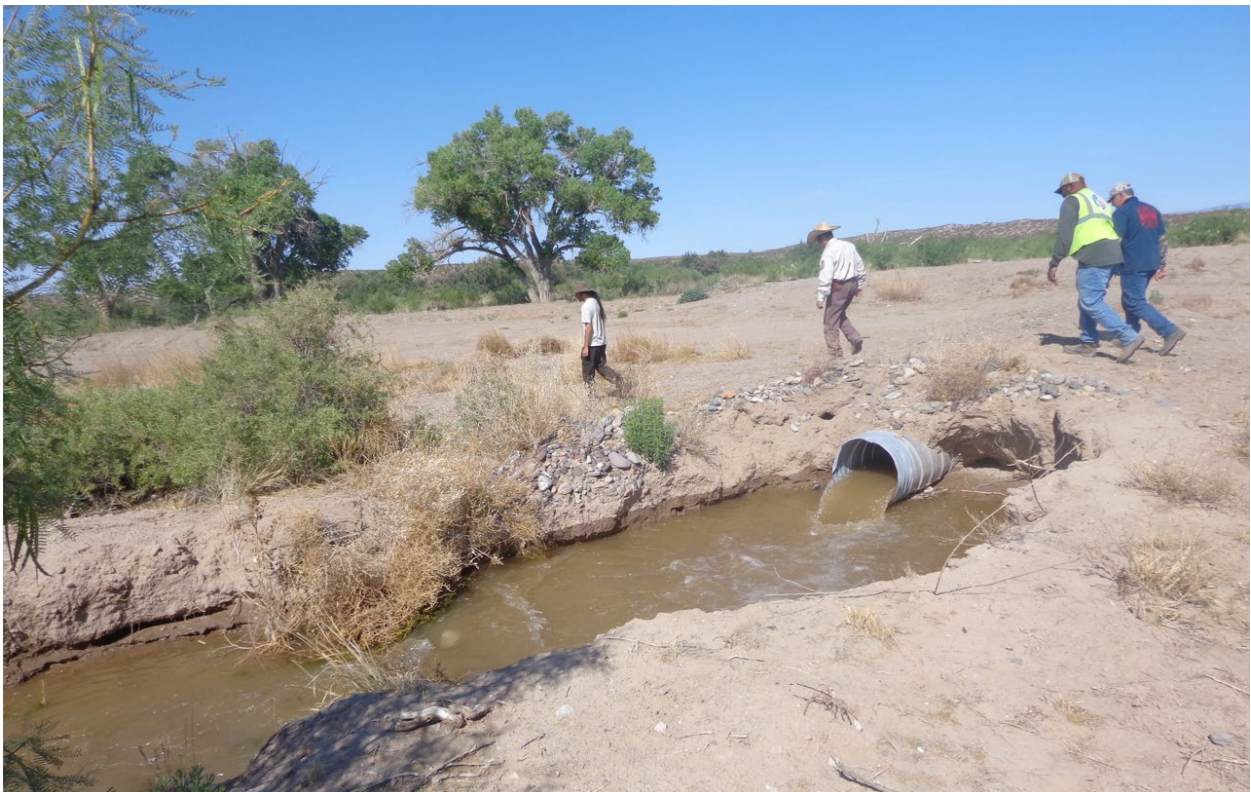
USFWS and USIBWC crews met at the site during the irrigation to discuss logistics of irrigations. Here, the water spills from the new culvert off of the Palmer Lateral into the excavated trench into the site.
