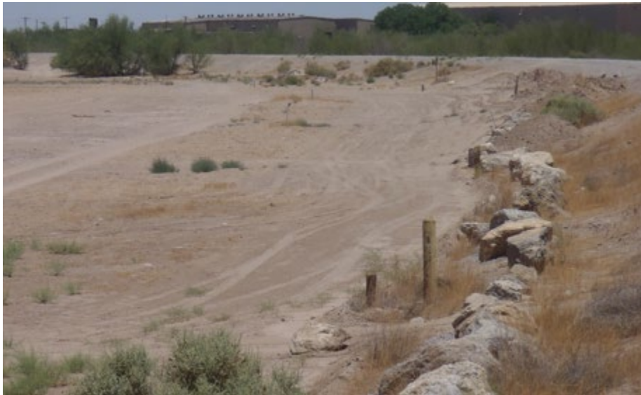
ATV/vehicle tracks up the landside of the west levee past the Vinton Bridge.
